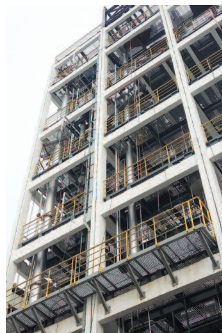
Figure 1: Distillation unit in Malaysia plant.
